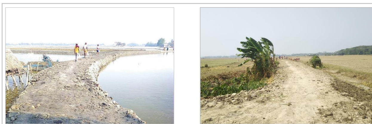
Figure 6: Earthen roads reconstructed through emergency employment supports in Lata Union under Paikgachha Upazila of Khulna (left) and Chandradeep Union under Bauphal Upazila of Patuakhali (right)
