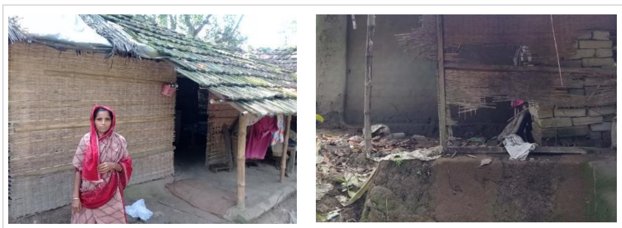
Figure 1: Fotema Begum, a beneficiary of Tayabpur village, Sarafpur Union under Dumuria Upazila of Khulna District with her repaired house (left) and damaged house before repair (right).
